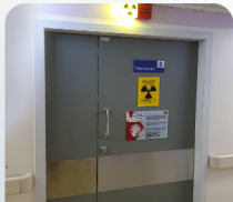
Lead Lined Door
